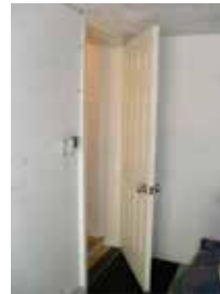
Left top: This steel garage-house door has no self-closing device
