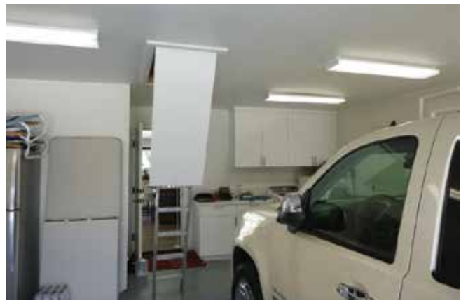
Non-rated pull-down installed in garage.
