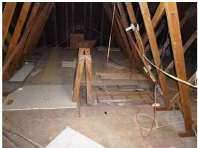
Non-rated pull-down installed in garage (same house as previous photo), as seen from the attic common to the house and garage.
