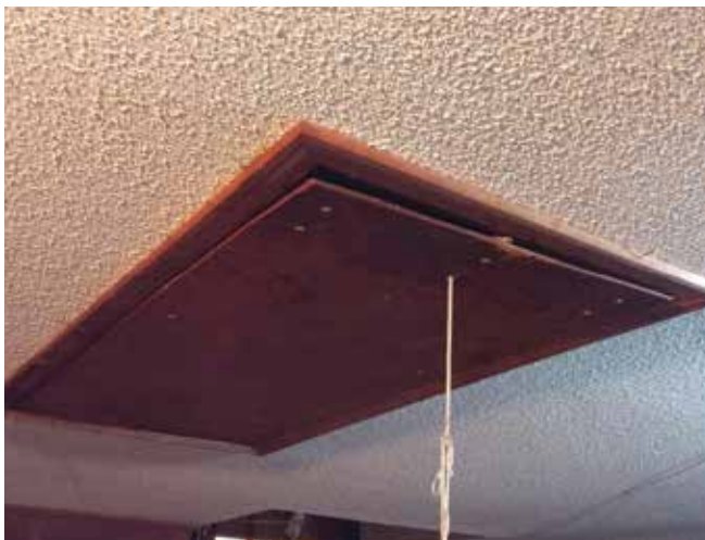
Non-rated pull down installed in a garage, with spring fatigue causing the door to sag when closed.
