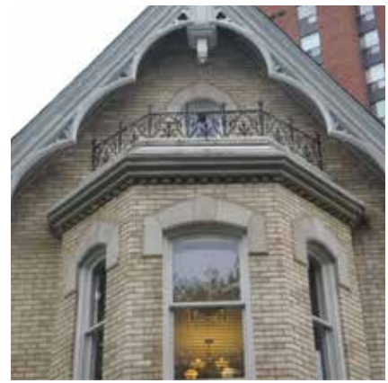
Here is an example of a Verge detail on a gable roof
