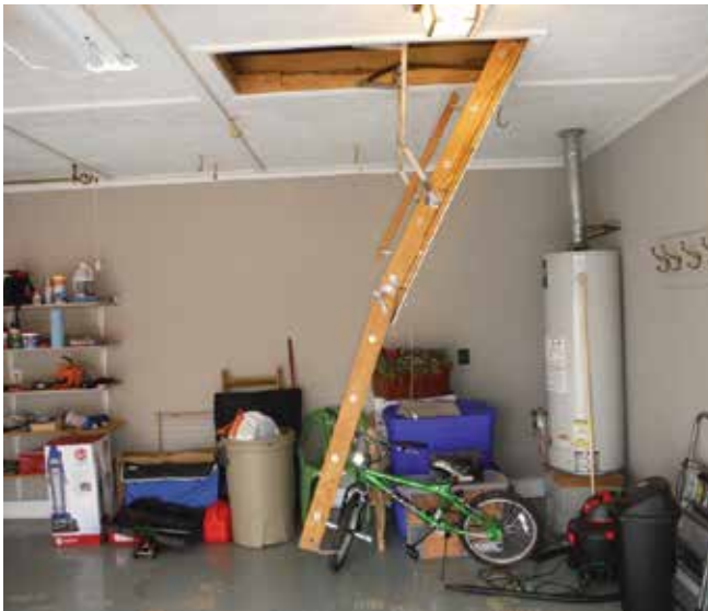
Attic stairs missing lower section
